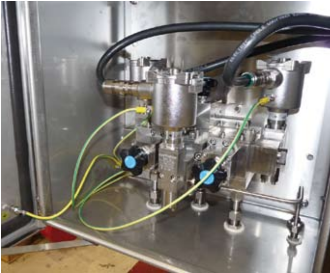
• Actuator control system
